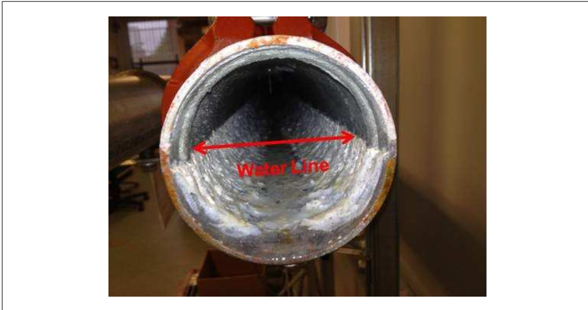
Fig. 4a. Galvanized steel pipe half-filled with tap water in house air after nearly six weeks' exposure
