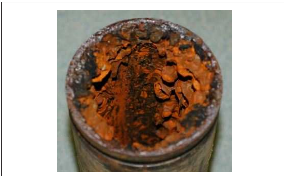
Fig. 15. Corroded steel pipe with many tubercles inside
