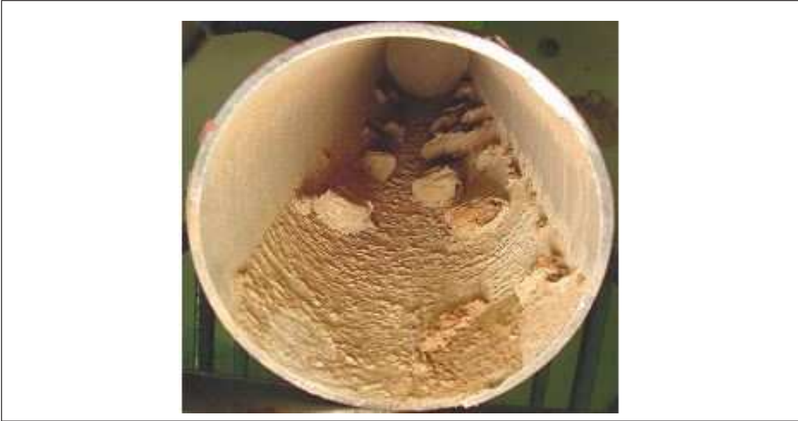
Fig. 9a. Tubercles that formed inside a galvanized steel sprinkler pipe (4 in. [10 cm] diameter)
