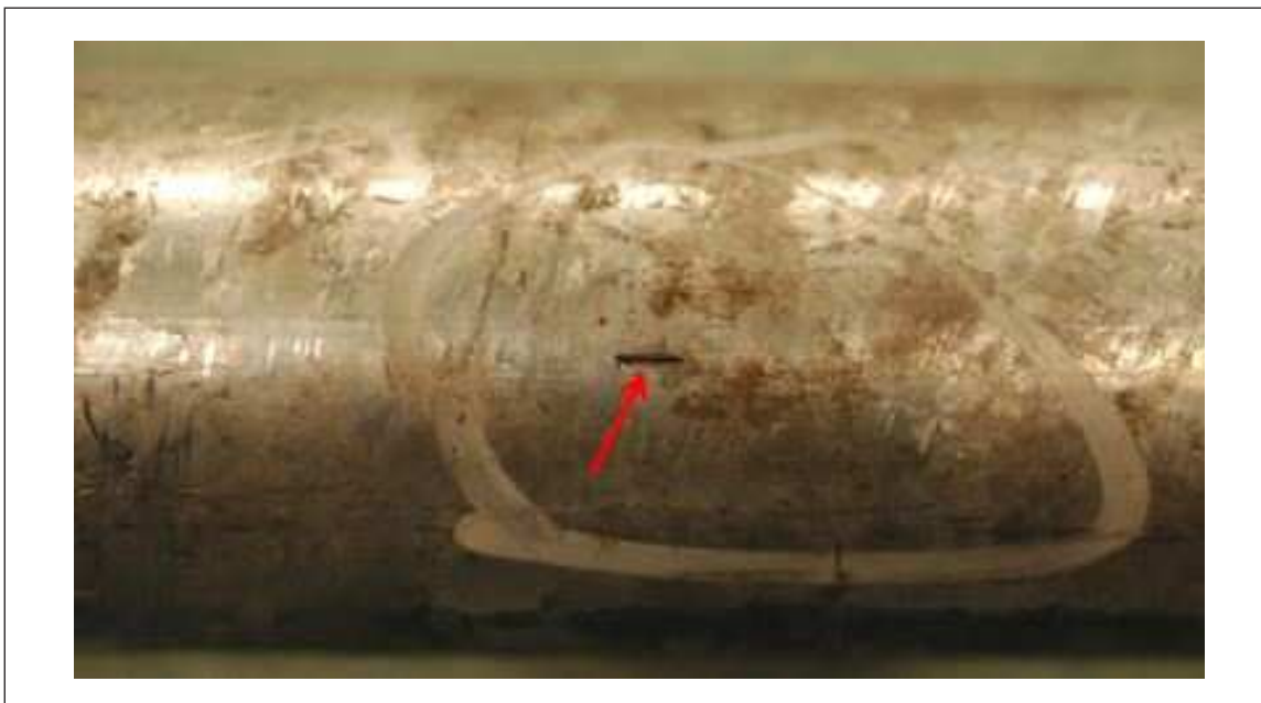
Fig. 14. Preferential grooving corrosion attack surrounding the weld seam area for a preaction system, near the pipe's 6 o'clock (bottom) installed position
