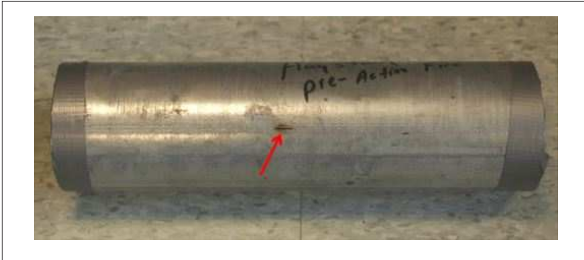
Fig. 13. Grooving corrosion of a longitudinal through-wall leakage in a galvanized steel pipe along its weld seam in a preaction
