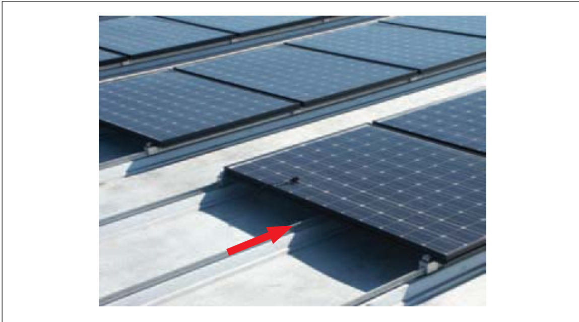
Fig. 3.2.2b. Unacceptable arrangement: clamp missing from SSR rib below middle of outer panel edge
