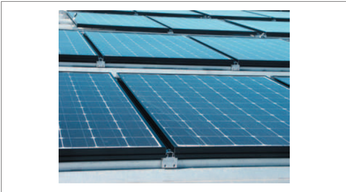
Fig. 3.2.2a. Solar panels secured to standing seam roofs using external seam clamps
