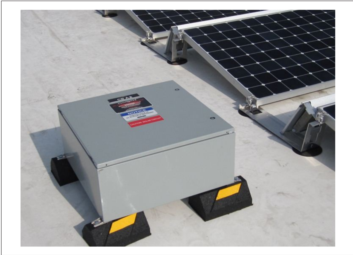
Fig. 3.2.1.1c. Equipment lacking anchorage to roof framing
