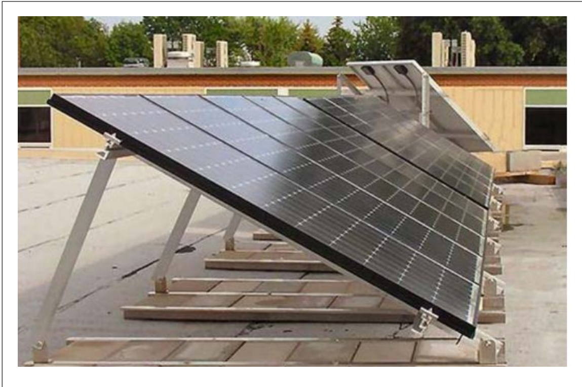
Fig. 3.2.1.1b. Solar panels with steeper slopes or lacking wind deflectors will experience greater wind effects
