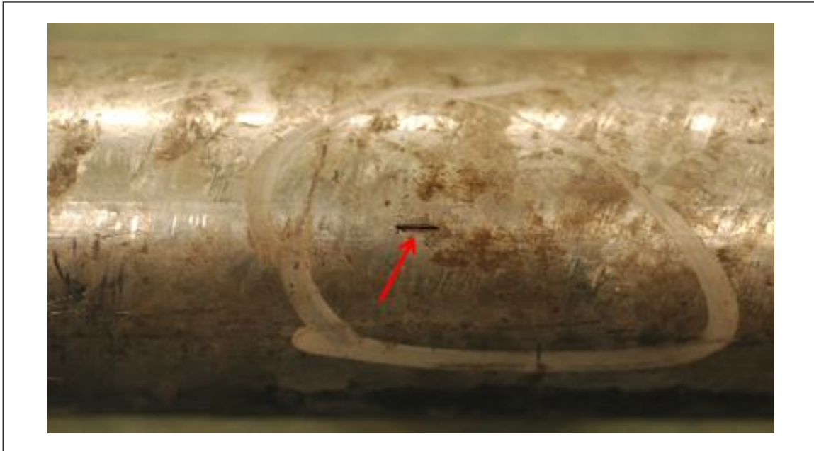
Fig. 14. Preferential grooving corrosion attack surrounding the weld seam area for a preaction system, near the pipe's 6 o'clock (bottom) installed position
