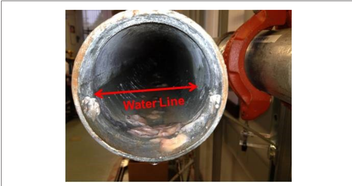
Fig. 4b. Galvanized steel pipe half-filled with compressed nitrogen after nearly six weeks' exposure
