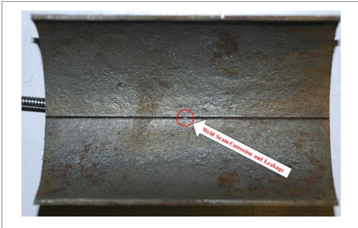
Fig. 12. Preferential grooving corrosion on a pipe weld seam with a .04 in. (1 mm) pinhole leak in a wet pipe system, after removing corrosion products inside an NPS 3 pipe
