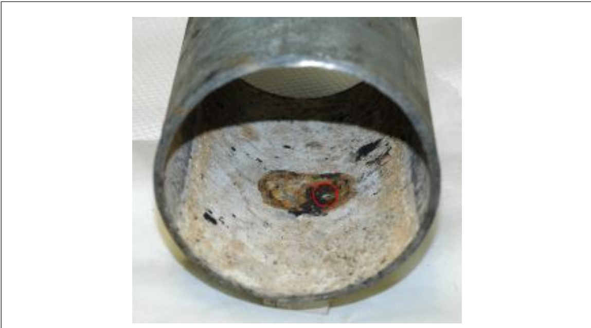
Fig. 9b. Corrosion at the base of a tubercle, which ultimately led to through-wall leakage
