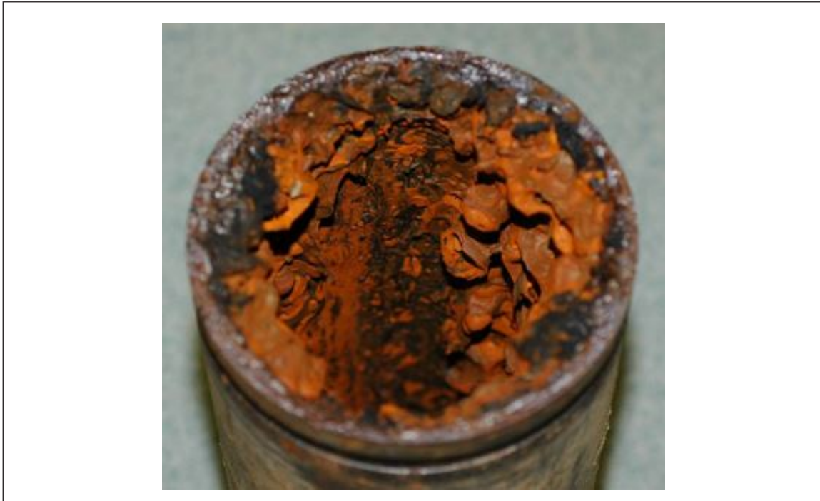
Fig. 15. Corroded steel pipe with many tubercles inside
